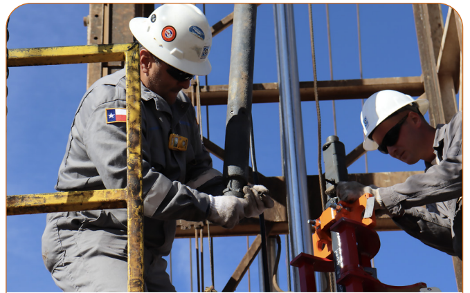
Field Service Technicians plugging in and securing the motor lead extension (MLE) to a permanent magnet motor during installation
